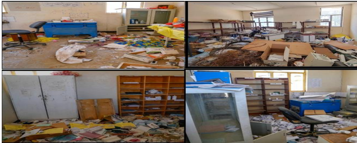
Figure 2.2. War damaged health facilities in kobo district. (Kobo town communication, 2023)
