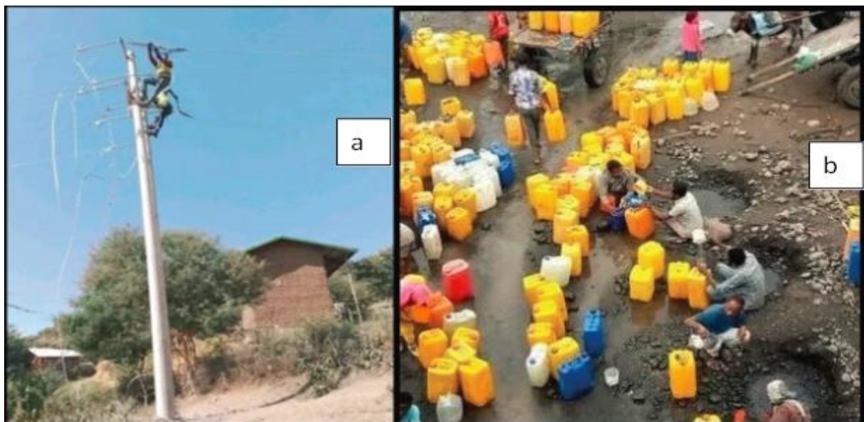
Figure 4.1. Overview of damaged infrastructure during the northeastern Ethiopian conflict (2021 – 2023). Note: a) Electricity technicians maintaining the war destroyed electric lines in NWE livelihood zone. b) Households from Gedober Kebelle fetching unsafe water from a nearby stream due to destruction of pipe water during the conflict.
