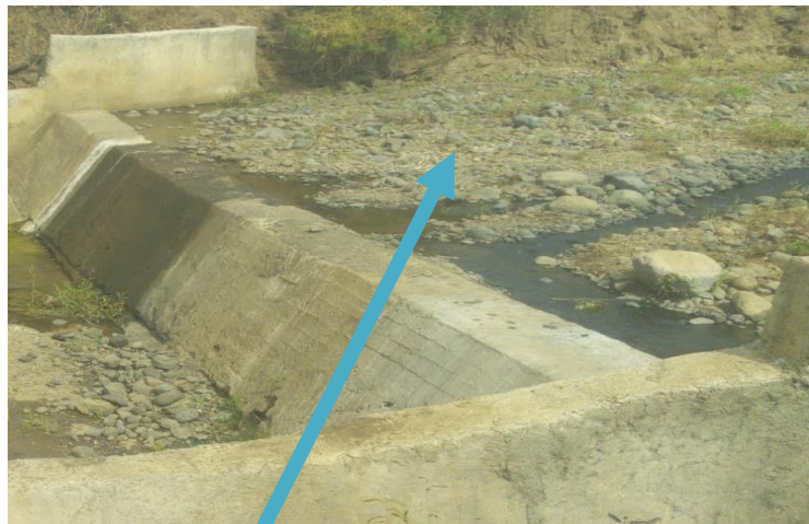
Figure 4-5 Siltation at head work
