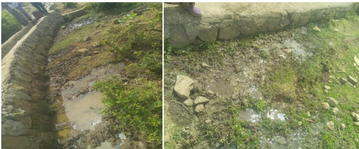
Figure 4-2 Seepage loss on the main canal
