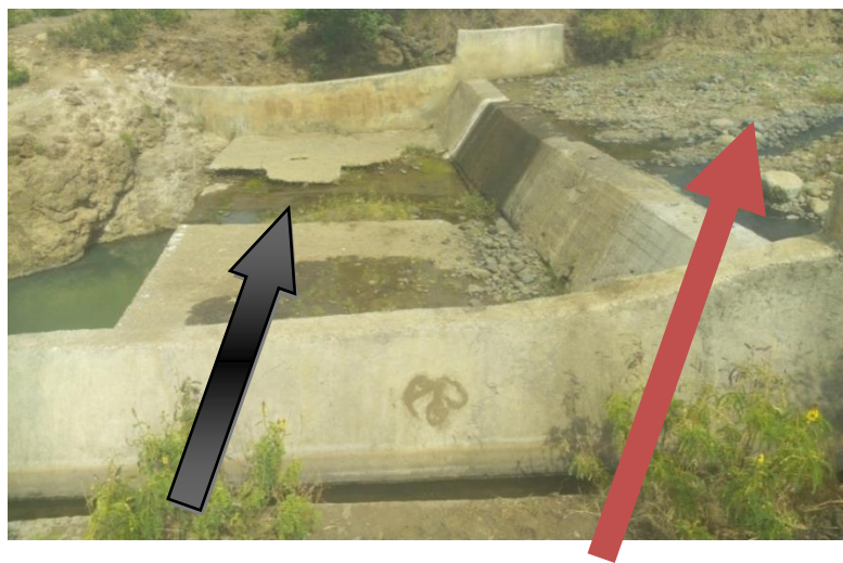
Figure 4-4 Flooding problem on apron structure and sediment accumulation
