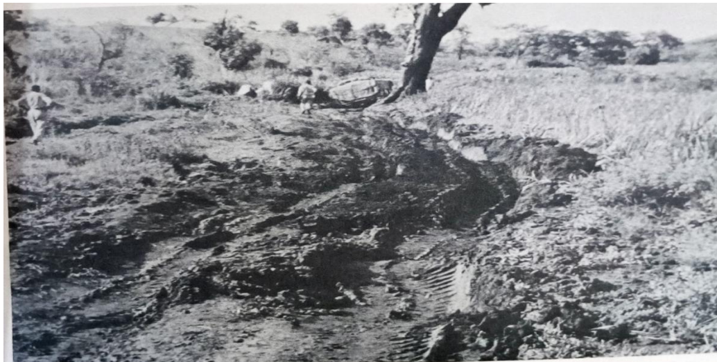
Figure 15: The deteriorated Bahir Dar-Dājān highway section, near Dājān. Source: Imperial Highway Authority Planning Team, Highway Construction in Ethiopia , P. 7.
