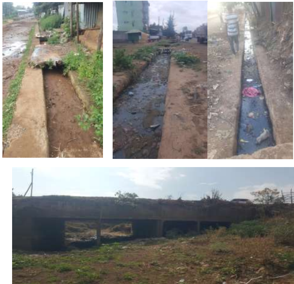
Figure 4.1 Observed existing conditions of some storm drainages and culverts in the study area
