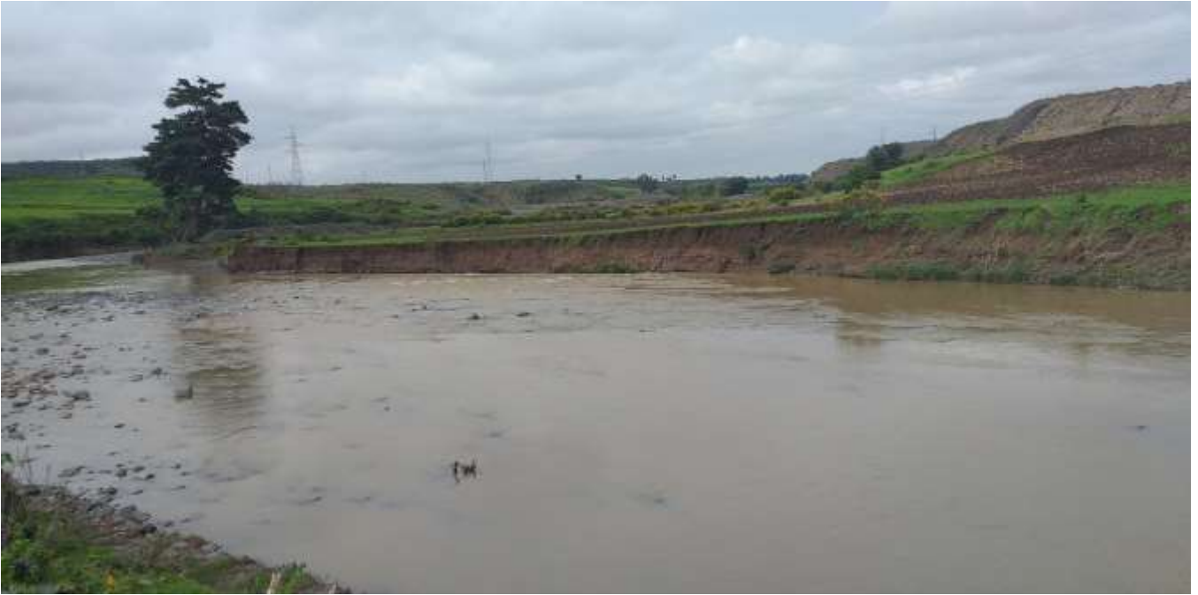
Figure 1: Megech River bank being widened by erosion: Taken from 200m downstream of Megech Dam, June 07/2019
