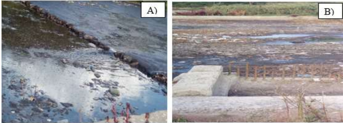
Figure 16: A) Drying bed cell's fractured common walls and B) accumulation of rubble and trash
