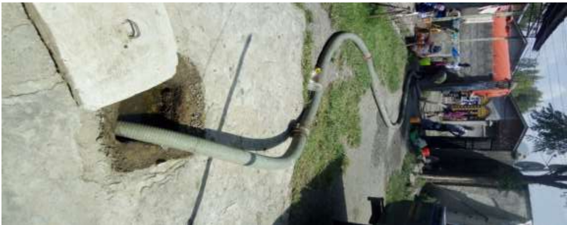
Figure 4.4c: Long hose from a municipal vacuum truck during fecal sludge emptying
