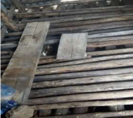
Figure 12a: Pit latrine with wood slab
