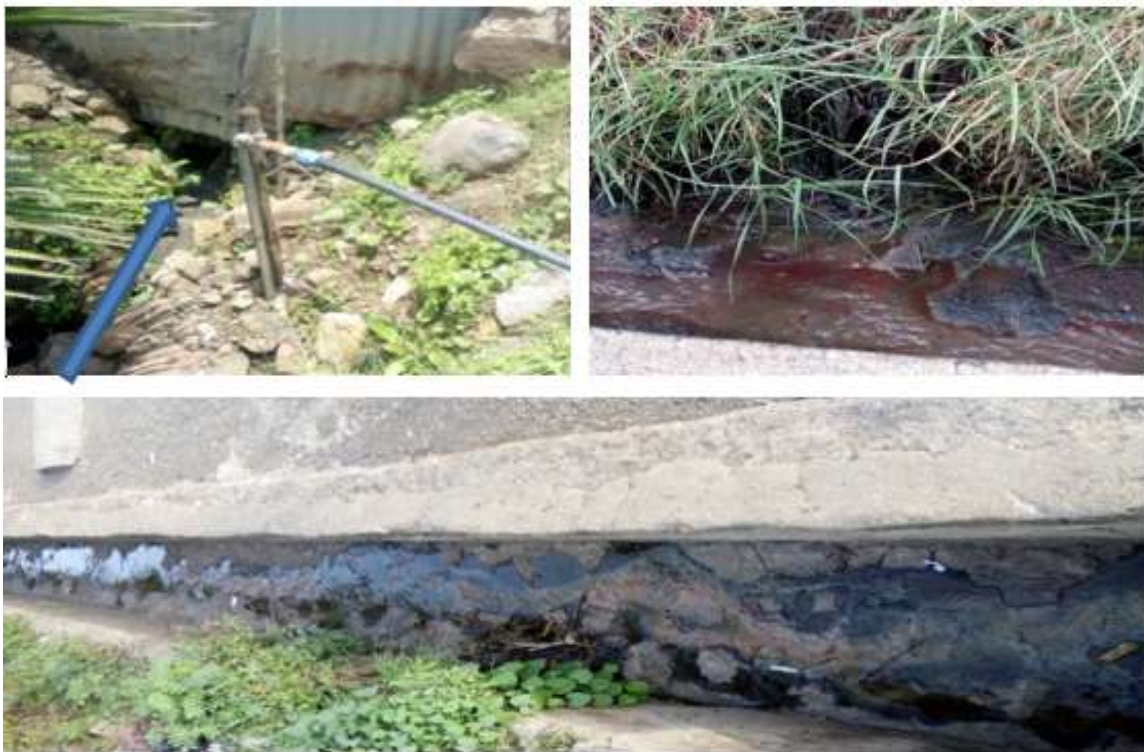
Figure 21: Illegal pit latrine and septic tank discharges through an open drain
