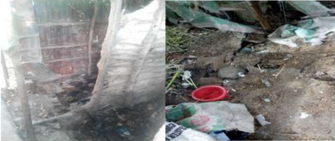
Figure 19: Collapsed pit latrine toilets
