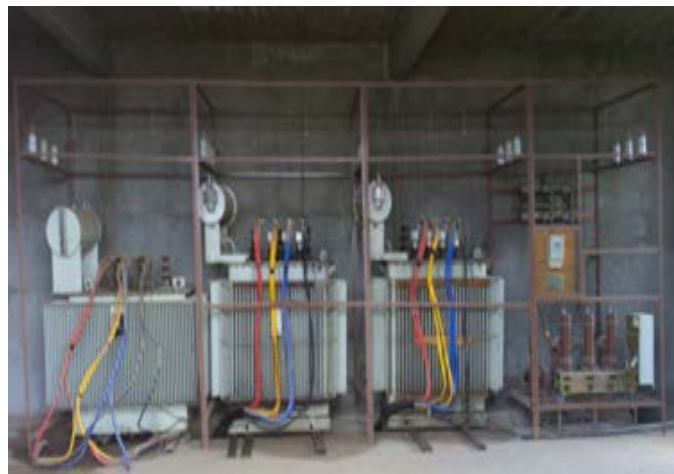
Figure 4. 2 Two 800KVA & one 1250KVA transformer
