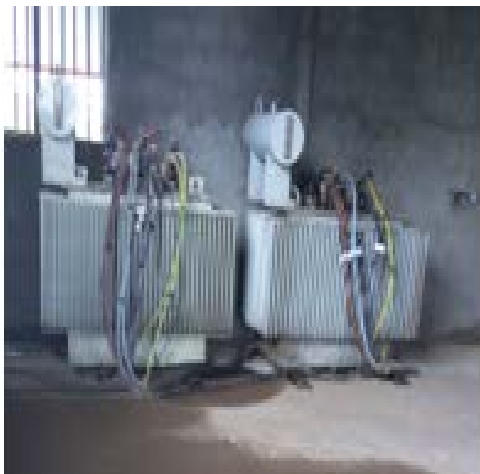
Figure 4. 1 Two 800KVA transformer
