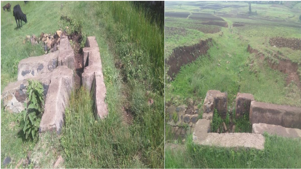
Figure 4.2 Nonfunctional division box
