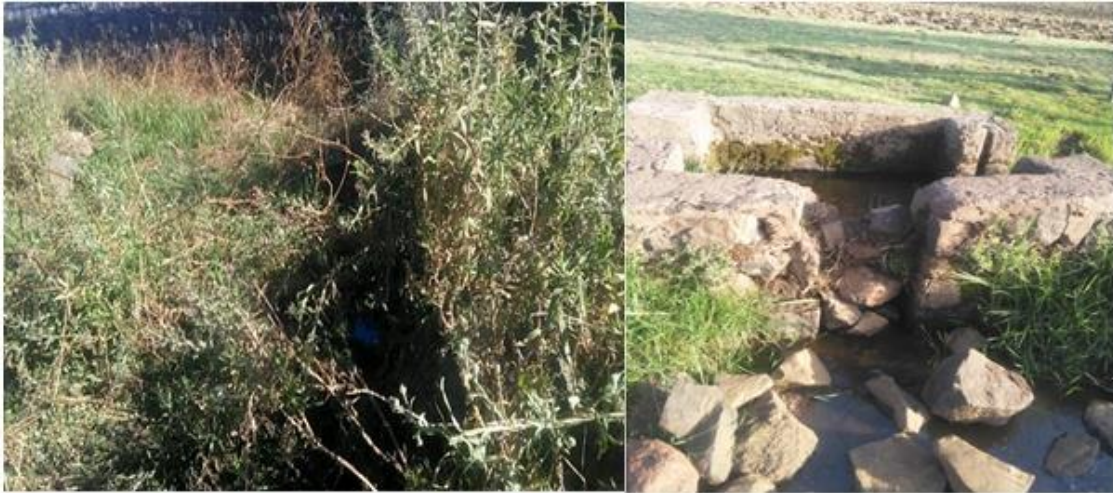
Appendix figure 3.5 Seepage and linkage problems.
