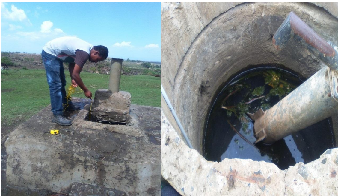
Figure 9: The abandoned groundwater table observation wells in the floodplain area.
