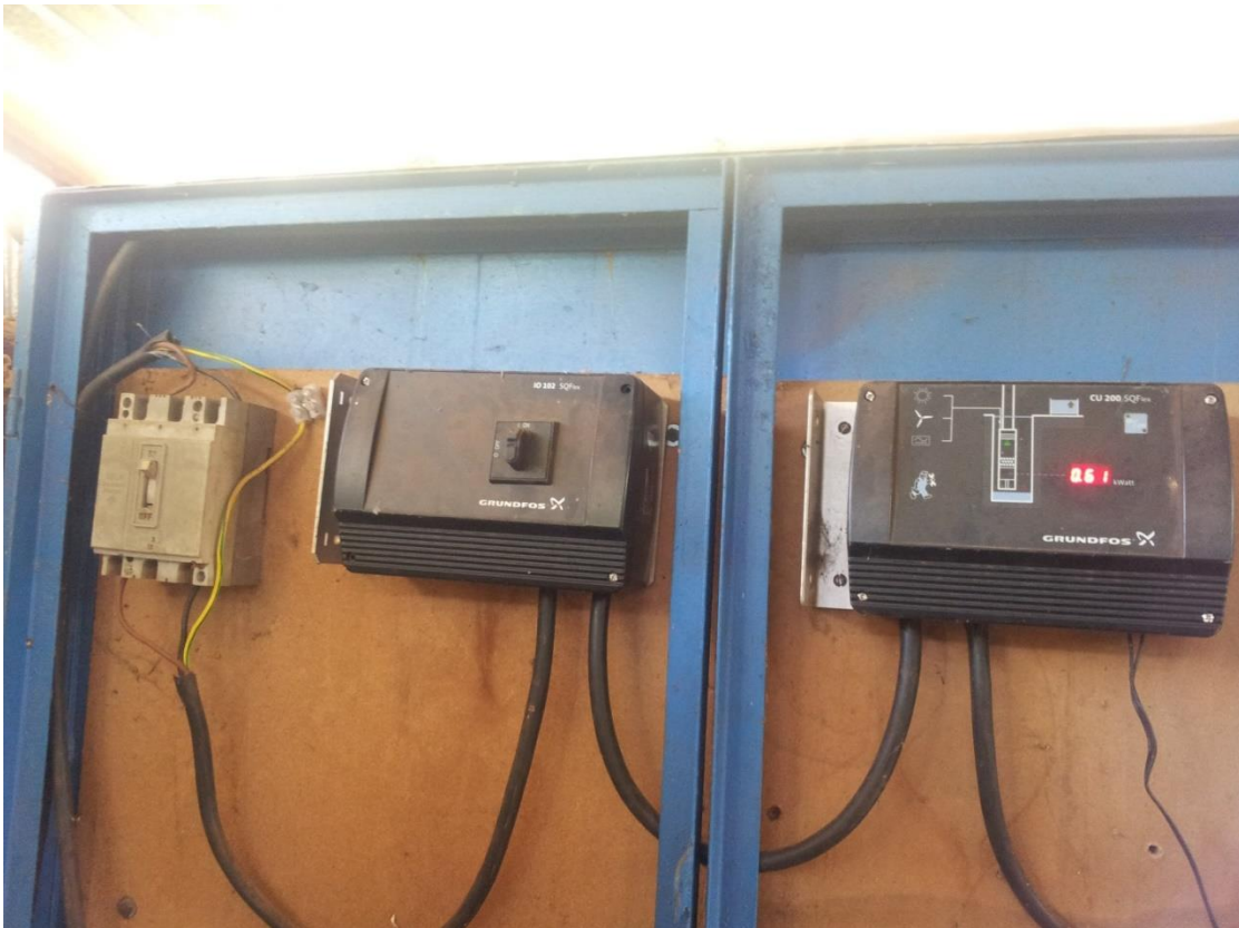
Figure 2.7: motor control board and breaker switch
