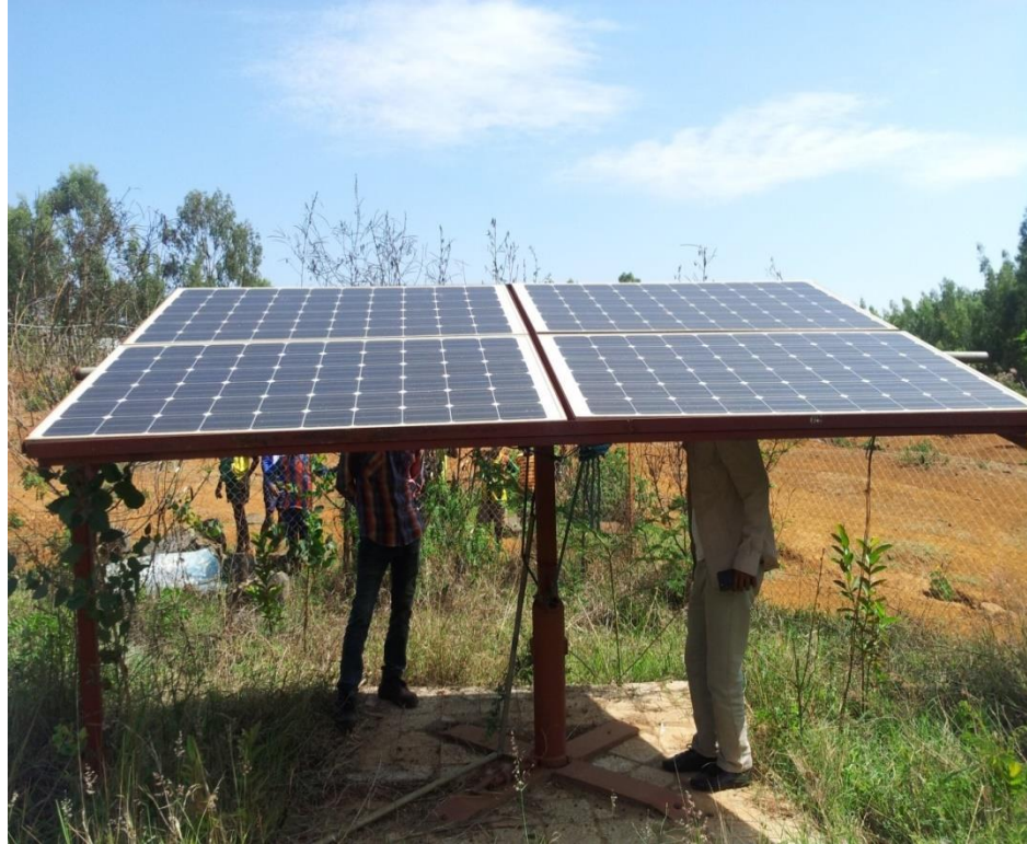
Figure 3.2: constructed solar panels installed at kolella keblel
