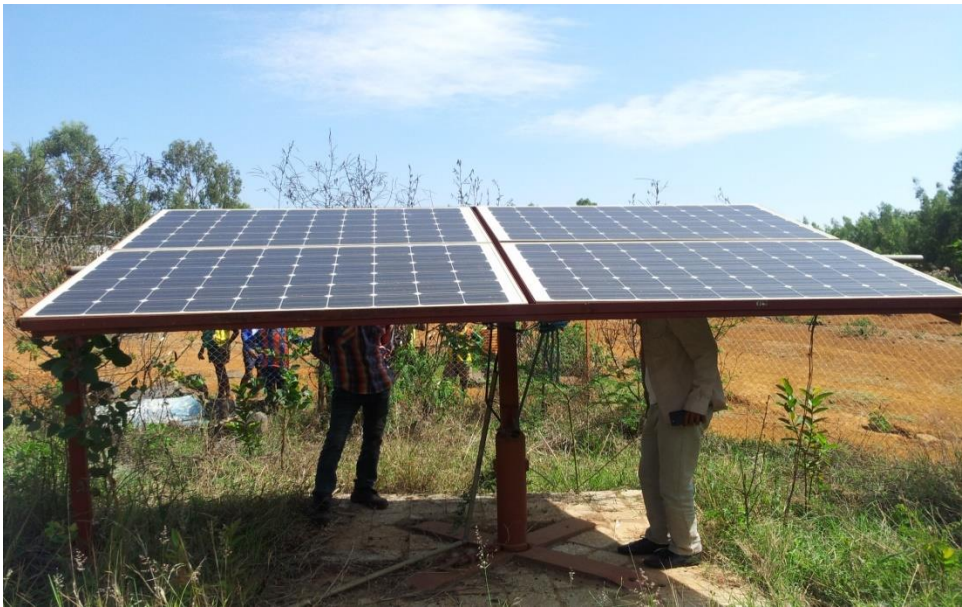
Photo of solar panel
